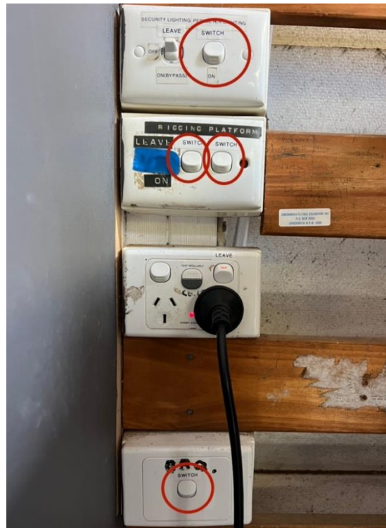
Detail of four (4) switches to turn off
